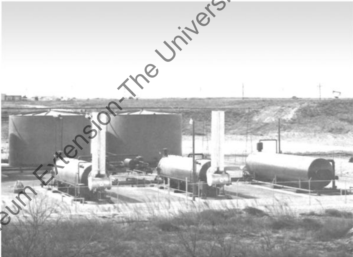
Figure 39. A central treating station with free-water knockout, electrostatic treaters, and stock tanks. A vapor recovery system, not visible, is also in use.
